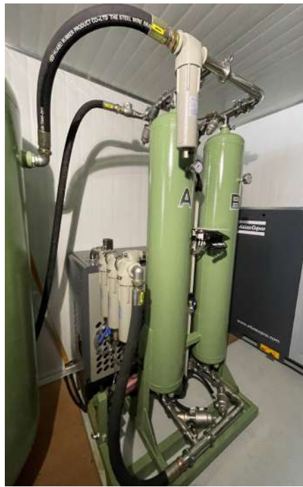
Freeze dryer and drying columns
