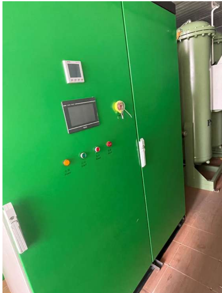
Container section with Ozone generator board and control panel
